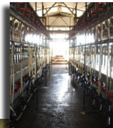
The Klein dairy has increased from a six to a 60 bail shed, producing significant amounts of effluent
